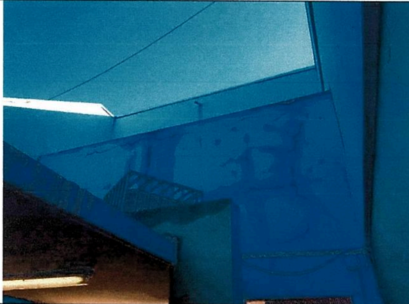
Picture 1 – Exterior CMU wall over main entrance beam has multiple horizontal and vertical cracks that go all the way through the wall section – Exterior View
