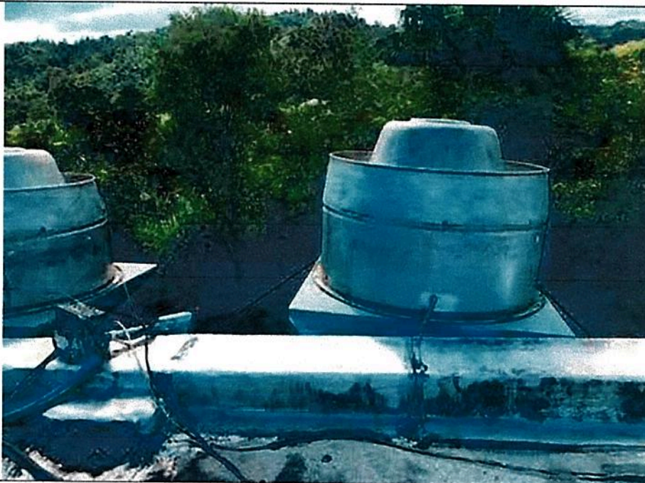
Picture 5 – Kitchen Ventilation Ductwork and Fans 2ea (Exterior) - Supports at roof level are extremely corroded and they are temporarily attached to the building by a coated wire with eye bolts. Both fan assemblies are wobbly.
