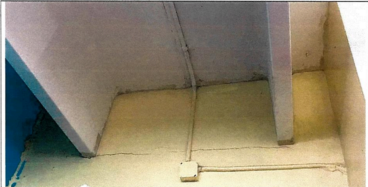
Picture 19 - Cracks (Horz.) between CMU walls and same CMU wall sections between each 2ble T Beam webs (many cases)
