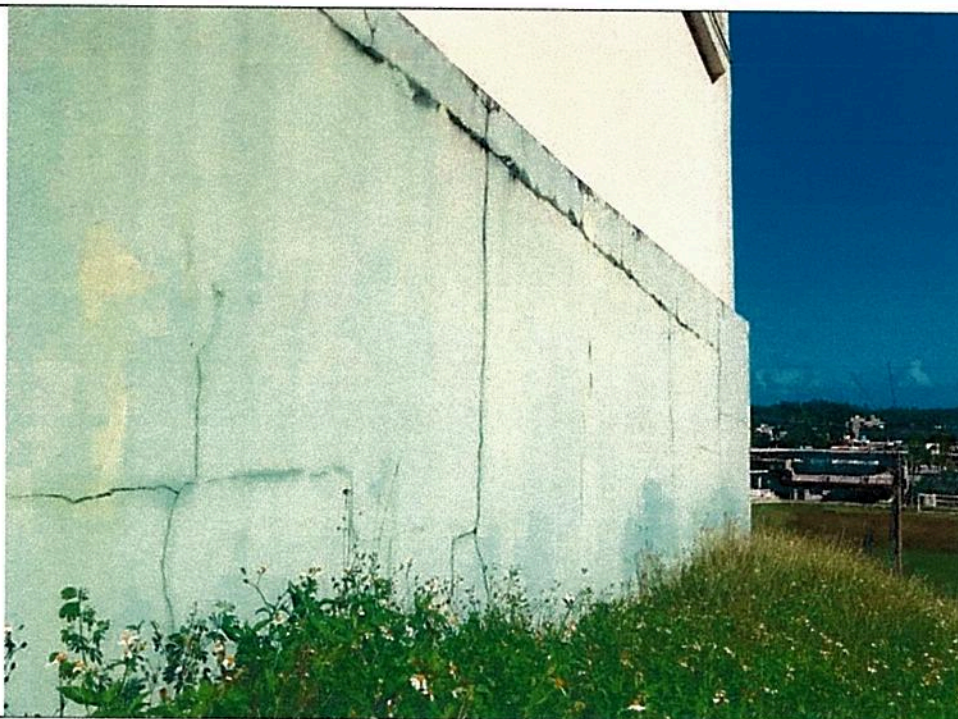
Picture 6 - Wide cracks (horizontal and vertical) at CMU wall under North-East part of the building. East side of the N-E corner.
