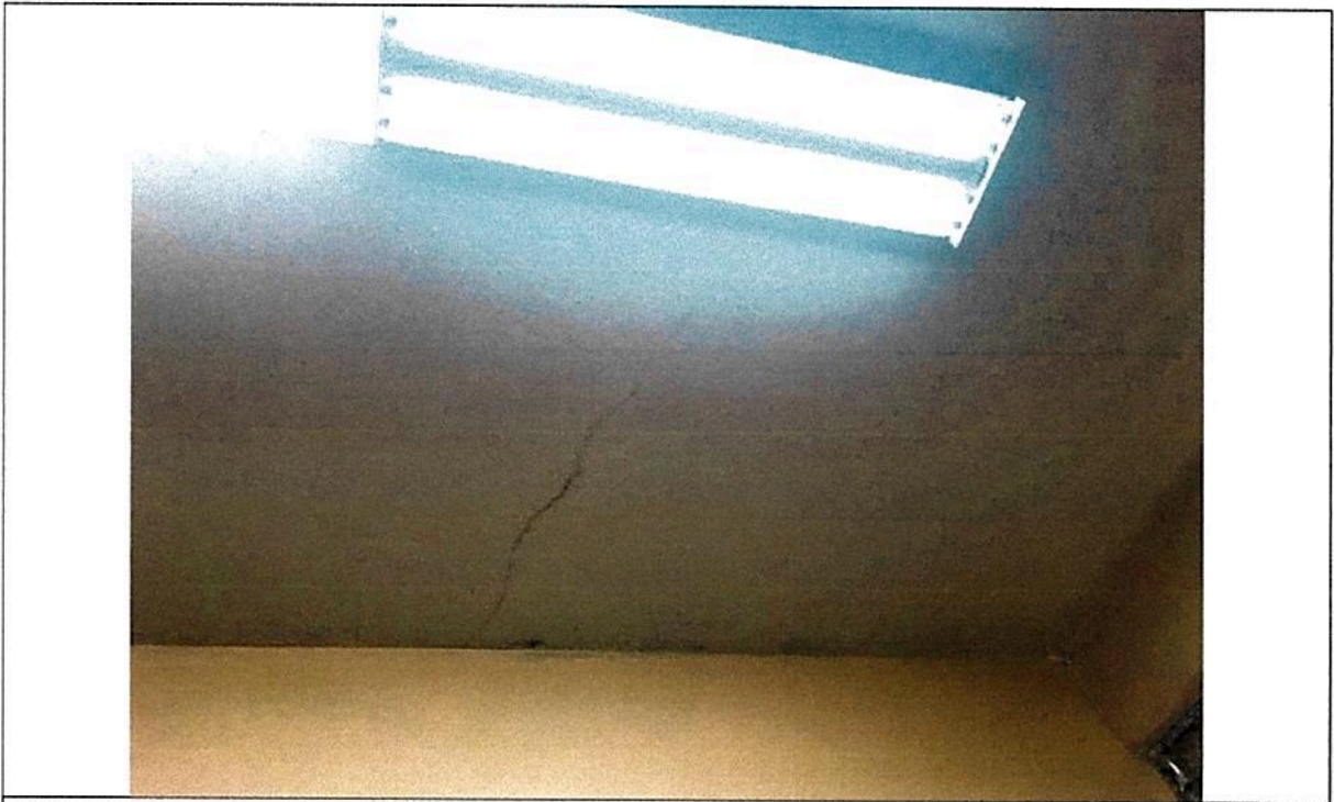
Picture 11 – Floor and roof slab cracks at the N-E building module (Classrooms)
