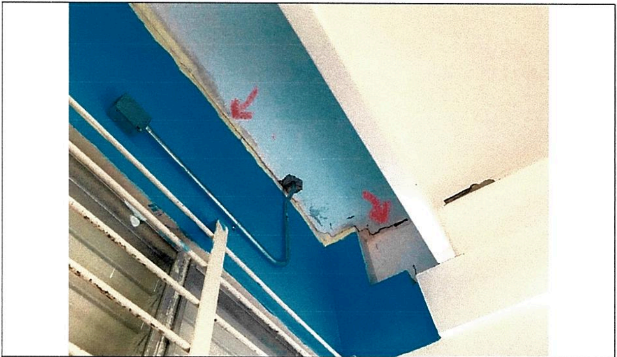
Picture 17 - Separations between 2ble T Beams' flanges and neighbor beams, walls and/or slabs. Delamination of finish plaster
