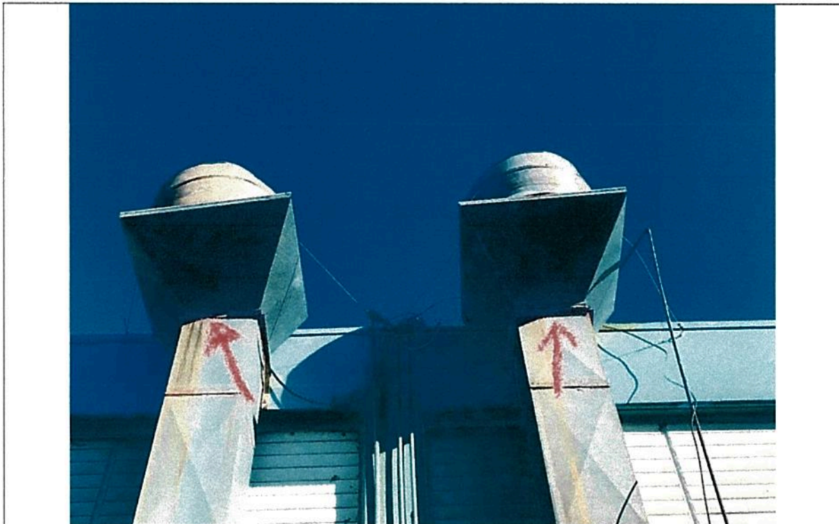
Picture 4 – Kitchen Ventilation Ductwork and Fans 2ea (Exterior) - Supports at roof level are extremely corroded and they are temporarily attached to the building by a coated wire with eye bolts.
